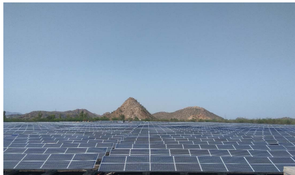
Hindustan Zinc Limited solar panels
