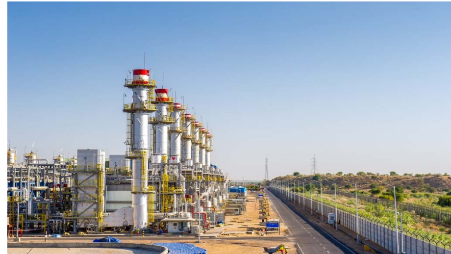
Rajasthan: Steam Turbine Generators at Mangala
